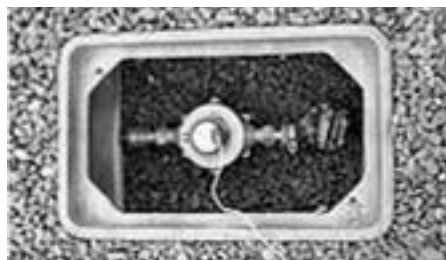
Typical meter installation
